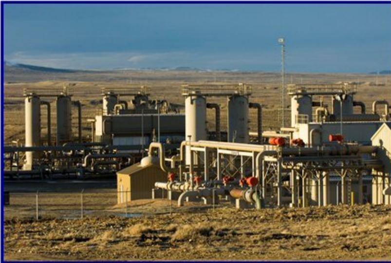
Pioneer Gas Processing Plant near Opal, WY
