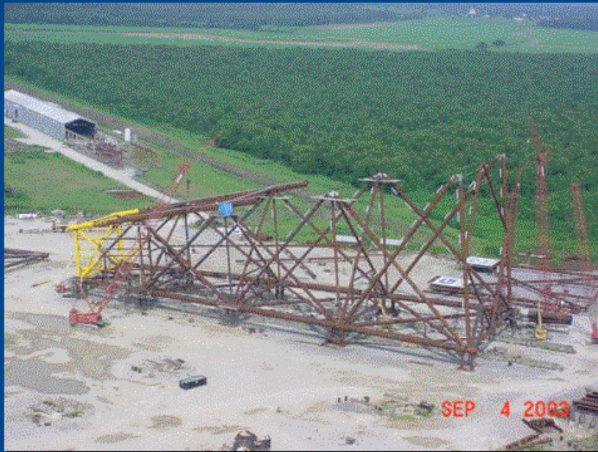
Fabrication of Ship Shoal 332 B Jacket at Gulf Island Fabricators, Houma, Louisiana
